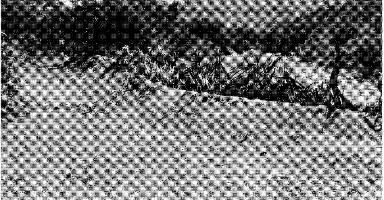
Figure 4.4. Water diversion structure on a tributary of the Rio Sonora near Baviacora, Sonora.
